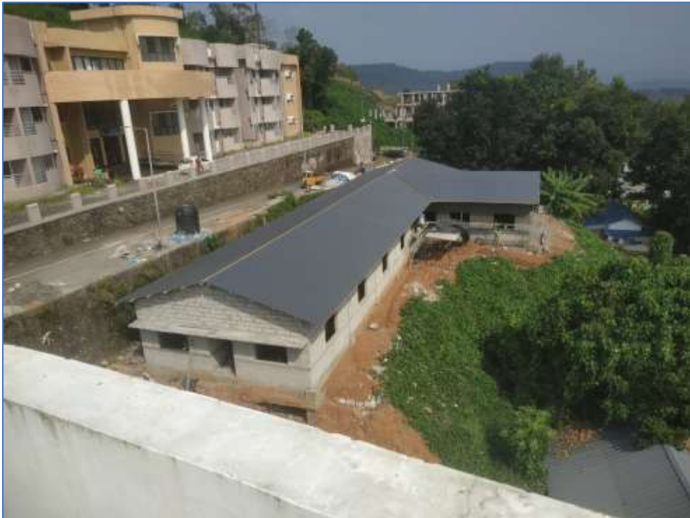
Single Storied Hostel for PhD scholars – Under construction - Through Internal Revenue Generation (IRG) (3 Jan 2023)
