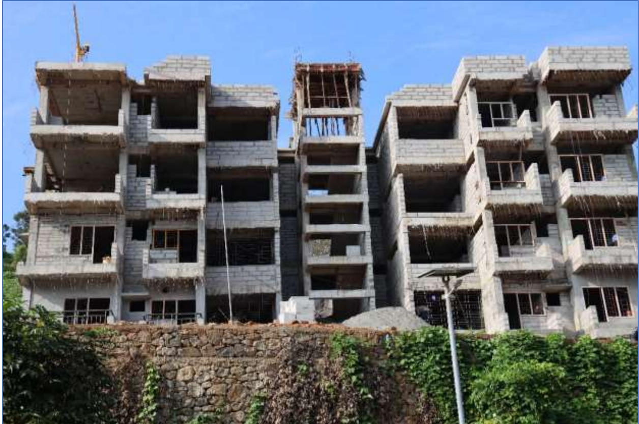
28 Staff Quarters 2 nd Building – Under Construction – Through Internal Revenue Generation (IRG) (on 05 Feb 2024)
