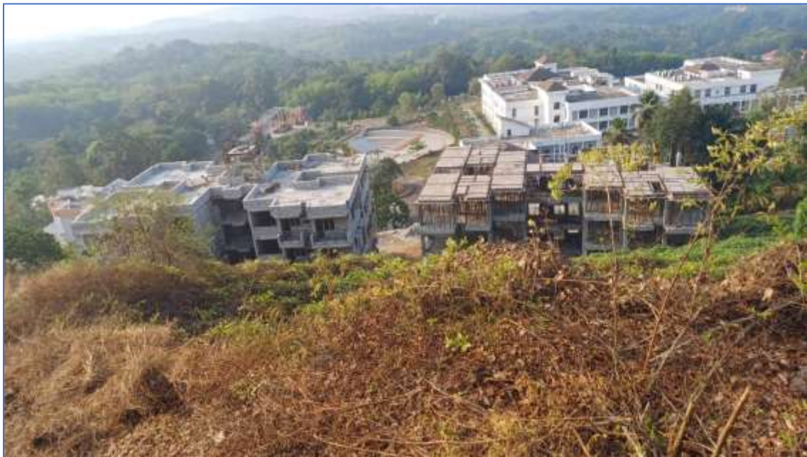
28 Staff Quarters Top View Both the Buildings– Under Construction – Through Internal Revenue Generation (IRG) (on 27 Feb 2024)
