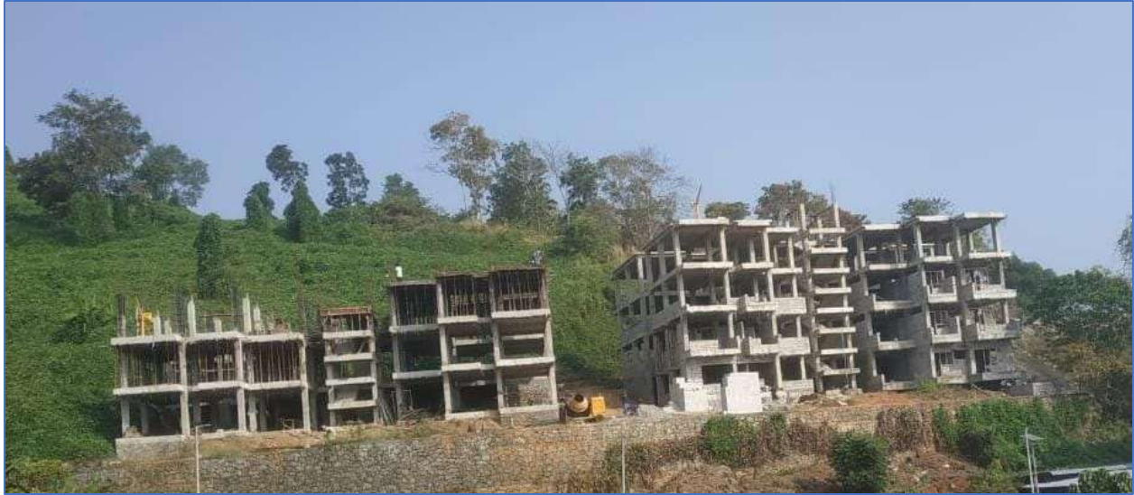
28 Staff Quarters Both the Buildings– Under Construction – Through Internal Revenue Generation (IRG) (on 03 Jan 2023)
